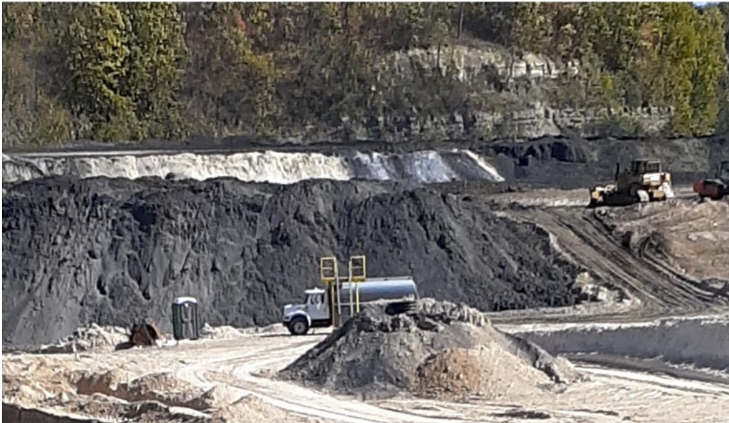
Photo 4 Typical view of leachate collection system riser pipe having a protective barrier surrounding the riser.
